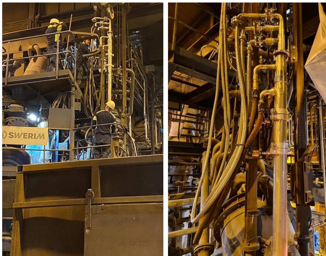
Figure 9. Installation of the CoJet lance at Swerim (left) and a close-up photo of the CoJet lance (right).
