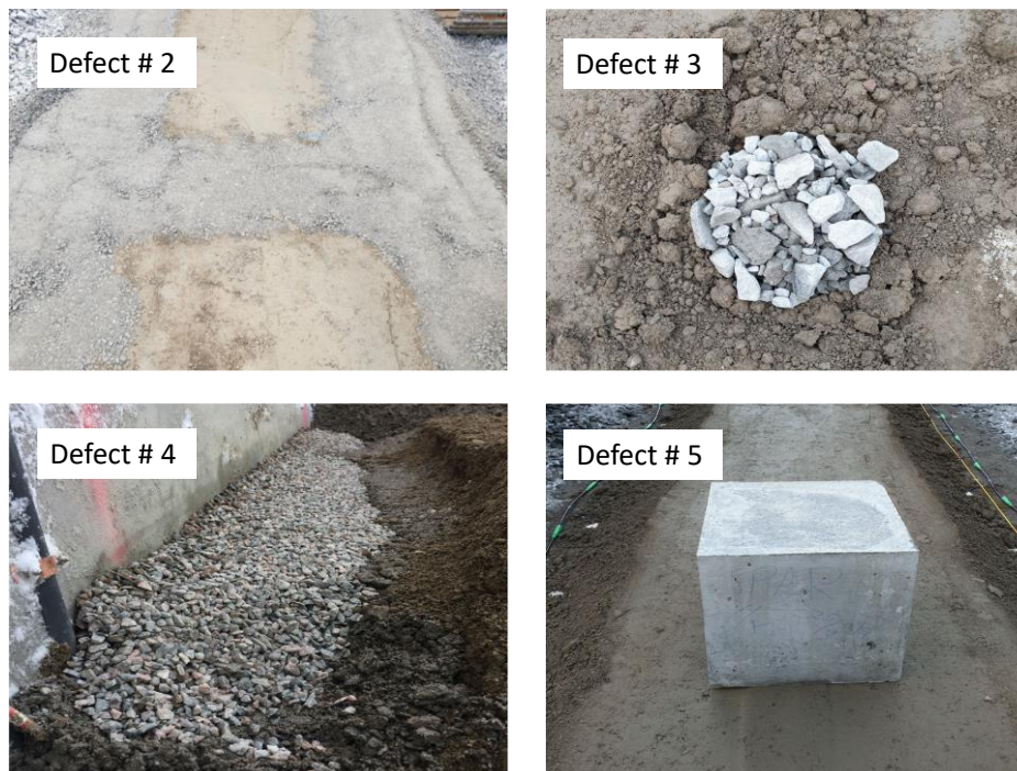
Figure 3 Description of the defects (Lagerlund et al., 2022).
