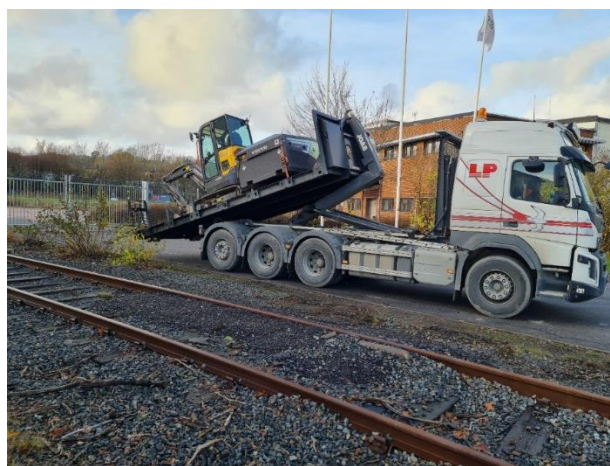
Figur 4 - ECR25 Electric & energilagrar, transport till site
