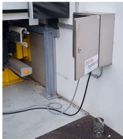
Semi-trailer connected to the gate
