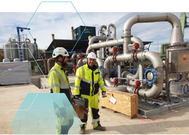
Figure 15. Project W4W – cost-competitive and grid-compliant biomethane from landfill gas using the WAGABOX® technology implemented in one of the largest landfills in Spain.
